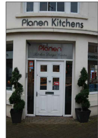
Schedule of Dilapidation's Ref No. 4 Clause No 5.4 Cracking in stone ledge over ground floor shop entrance to be repaired ready for redecoration
