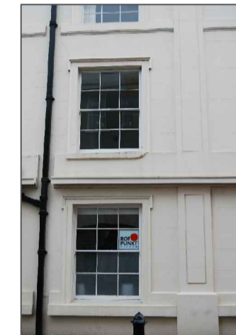
Repair existing window cill to first floor west elevation ready for redecoration
