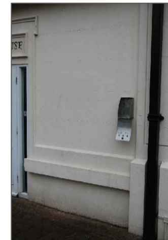
Schedule of Dilapidation's Ref No. 3 Clause No 5.5.2 Remove cigarette bin, fill and repair fixing holes ready for redecoration
