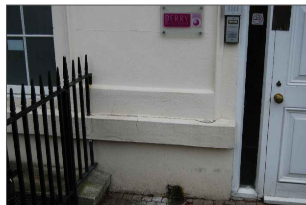
Schedule of Dilapidation's Ref No. 8 Clause No 5.4 Low level stone ledge to left hand side of ground floor office entrance door is displaying signs of cracking. Contractor to investigate cracking and repair cill. Make good cill ready for redecoration.
